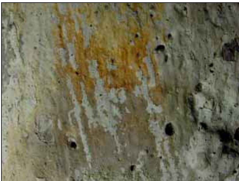
Below: Detail from the north side of the Crucifixion showing that the yellowish secondary paint has been covered by a layer of whitewash
