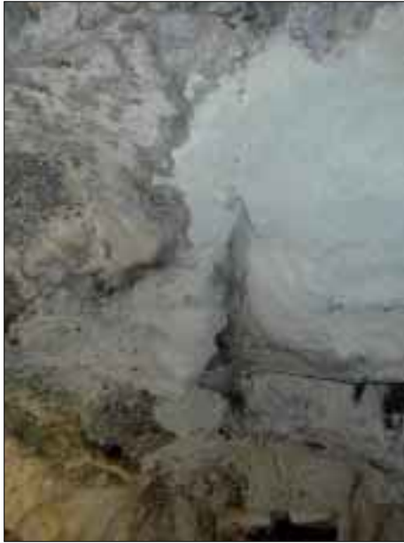
Crack between basalt blocks in the roof of the chapel. Location of photo, appendix 1, no. A
